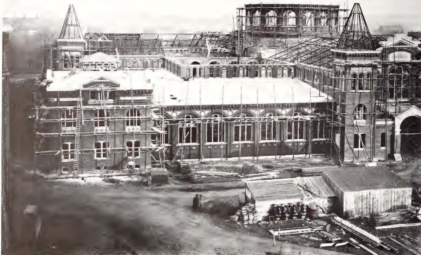
United States National Museum under construction, probably in 1880. The picture was taken from the Castle, looking east toward the Capitol.
